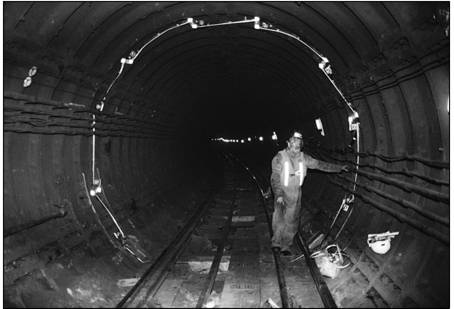
Dr. Richard Bassett installing the original BCS in a London Underground tunnel.
