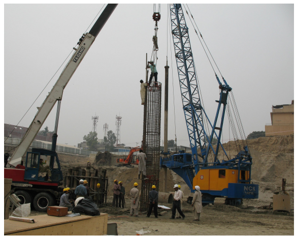
Above Left : The top section of the cage is lowered onto the bottom and fixed together, The technicians stand next to the cage ready to install four sister bars at the point where both reinforcement cages are joined.
