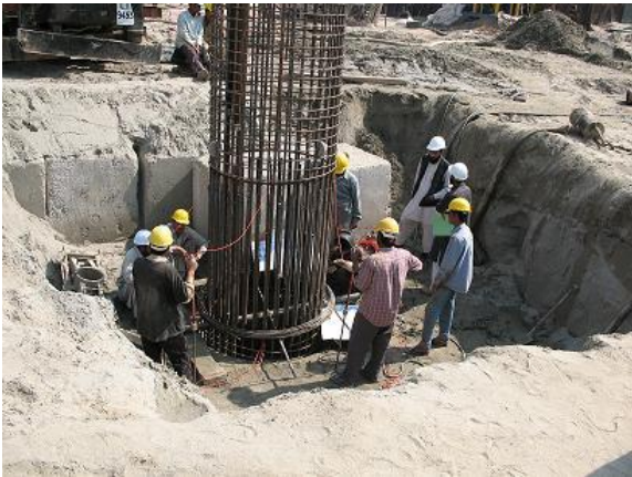
Above right : The bottom section is suspended at the top of the borehole so that the top half of the cage can be positioned and joined.
